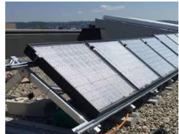
Roof top PV
